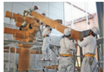
The process of assembling a model bracket complex of Toshodaiji Temple was disclosed in the commemorating traveling exhibition, " Toryo —the world of temple and shrine carpenters."
