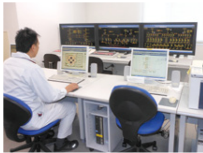
Service provided at the facilities' central monitoring room
