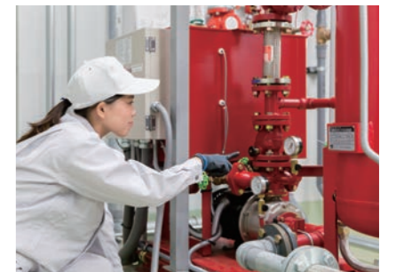
Daily facilities check
