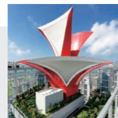
A large air intake ("funnel") as high as 45 meters is installed on the rooftop garden to supply fresh air, which is cleaner than the air closer to the ground, to each office in the building.
