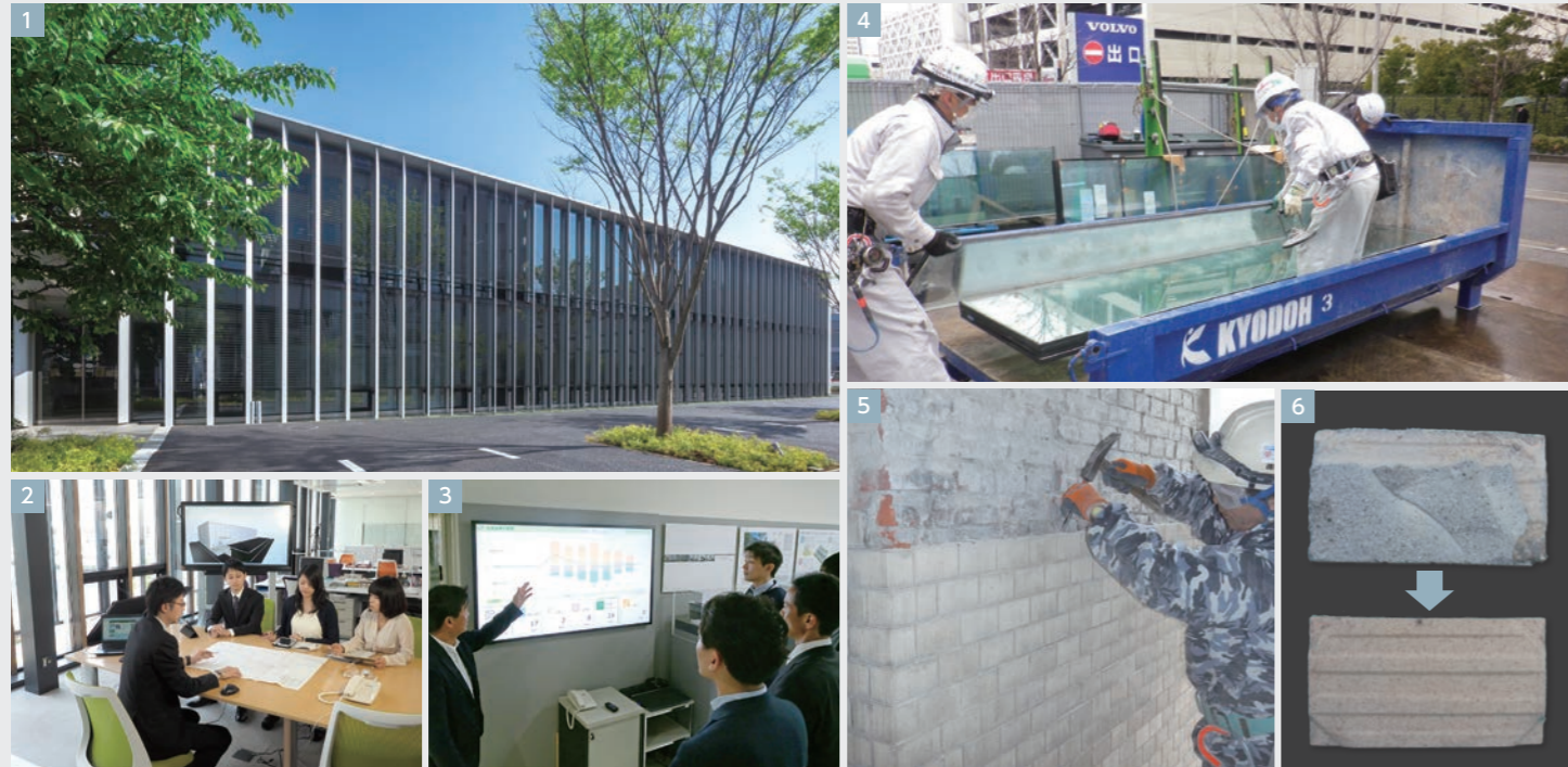
1. Outer appearance of the Higashi Kanto Branch Office building after renovation into a ZEB 2. The communication area provides different types of work spaces that can be selected according to purpose 3. Displays energy balance in real time 4. Replacement, separation and discharge of glass (a ZEB project at the Higashi Kanto Branch Office) 5. Chipping work for recycling and reusing tiles (KITAKARO Sapporo Honkan site) 6. Top: A tile before removing mortar Bottom: A tile after removing mortar
