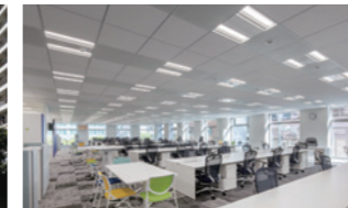
DC power LED lighting in the Kurihara Kogyo Building in Kita-Ku, Osaka Prefecture
