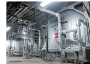
Methane fermentation tank on a basement floor of Abeno Harukas
