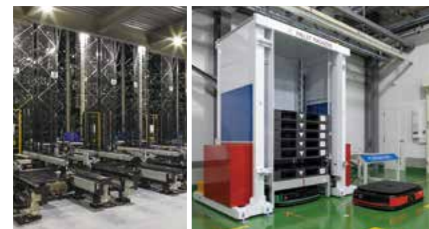
Automated storage/distribution system (right and left)
