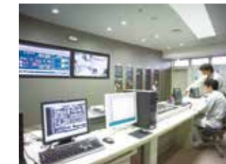
Centralized facility monitoring
