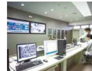
Centralized facility monitoring
