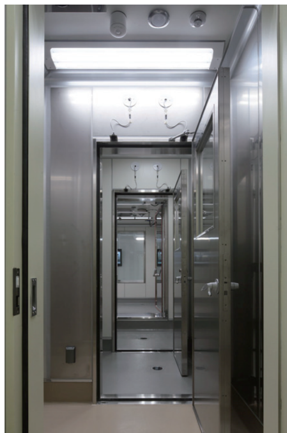
Photo 8 様々な内装仕様で構成された前室 Pass-rooms which consists of the various interior specifications
