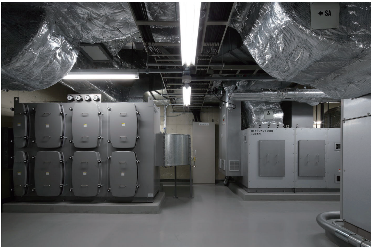
Photo 3 B1F 空調機械室 B1F air-conditioning machine room
