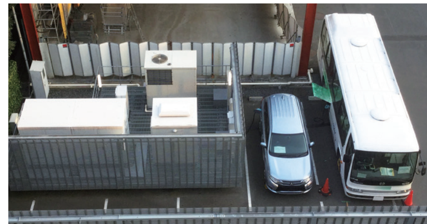
Providing electricity to a building for more than 72 hours from 2 PHVs
