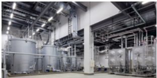
Cooking oil tank room (cooking oil supply equipment)
