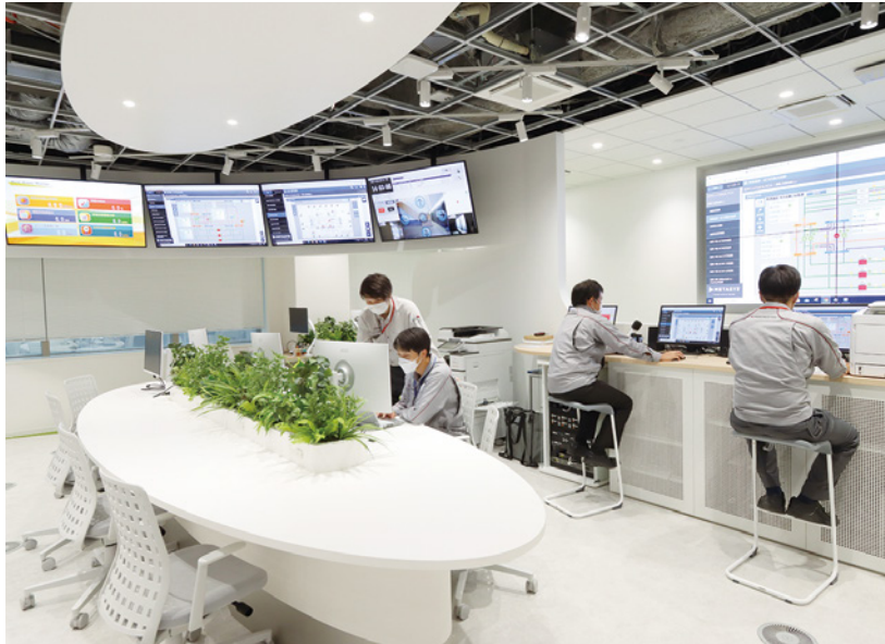
Centralized Control Center for next-generation building management
