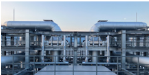
Rooftop equipment area (waste heat and wastewater recovery equipment)
