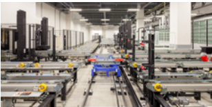
Shipping area (automated transport equipment)
