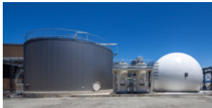
Environmental equipment area (methane fermentation equipment)
